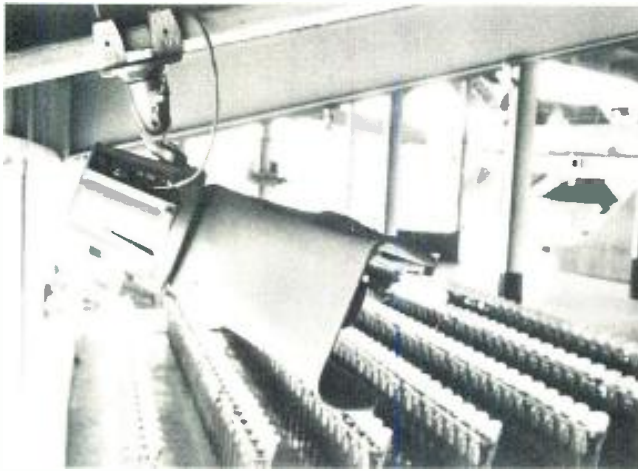
Double re-entrant projector speakers are mounted on support beams and ceilings with a three-way adjustable bracket.
