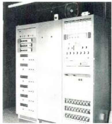
Located in the main control room, the fan-cooled control console incorporates an automatic lighted relay speaker network crossover (bottom right) for emergency transfer of speakers without dispersion loss in case of amplifier failure.
